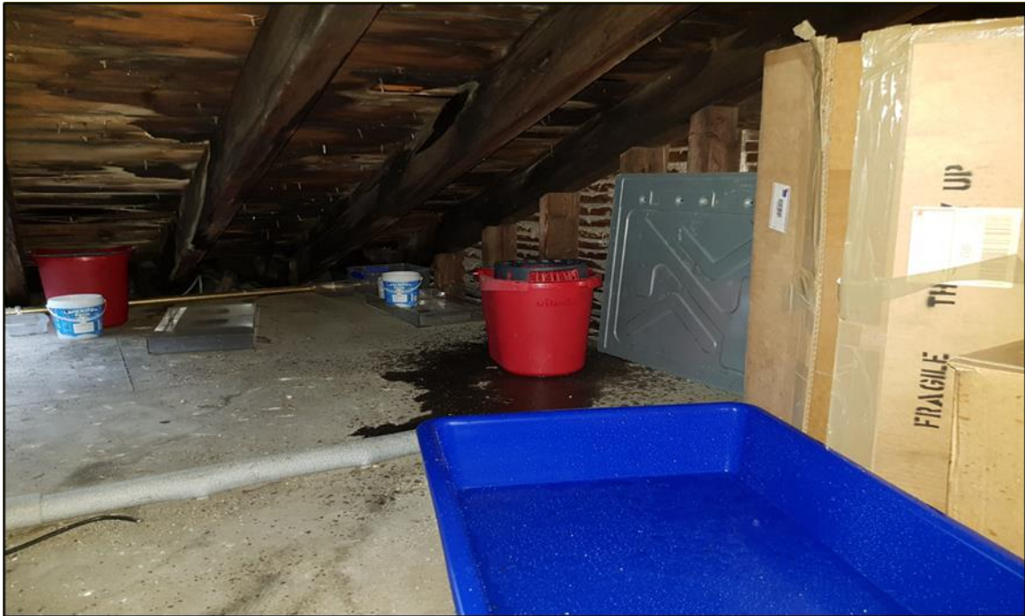
Figure 8: Buckets catching water from the leaking roof.
