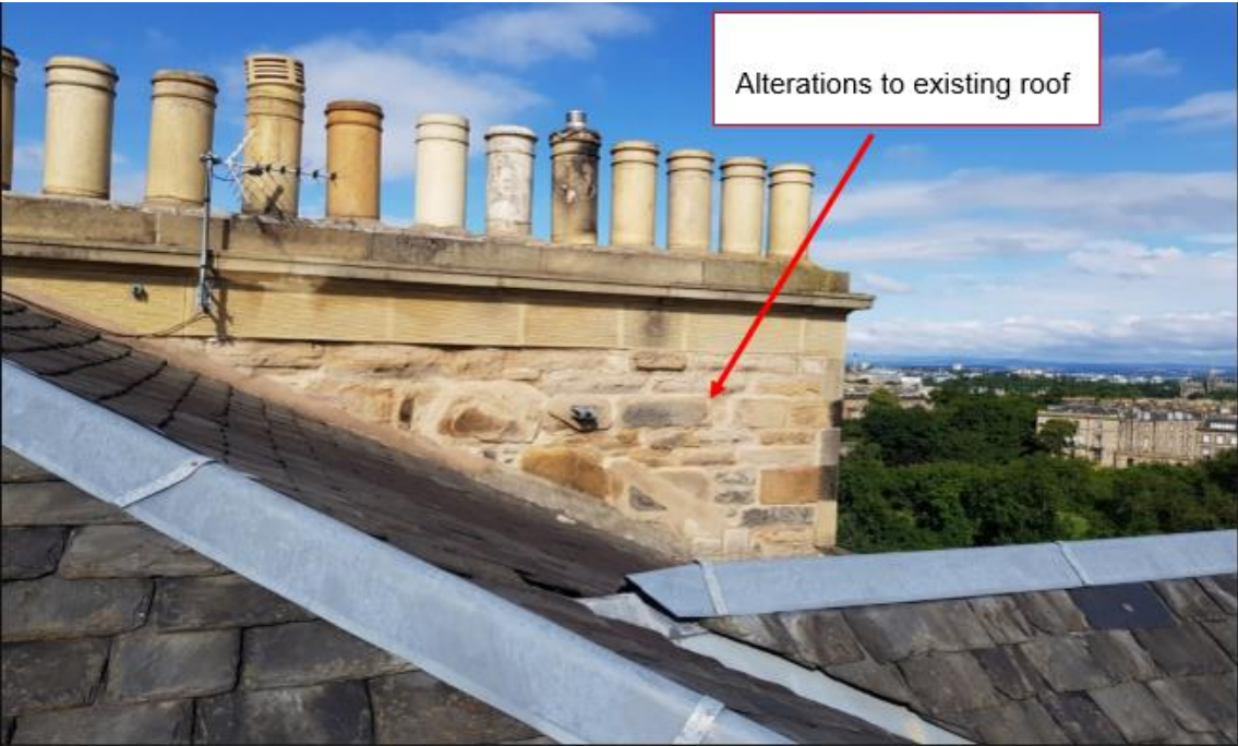
Figure 3: previous alterations to the original roof of no. 10 Randolph Crescent facing rear (north), as evidenced on chimney stack.
