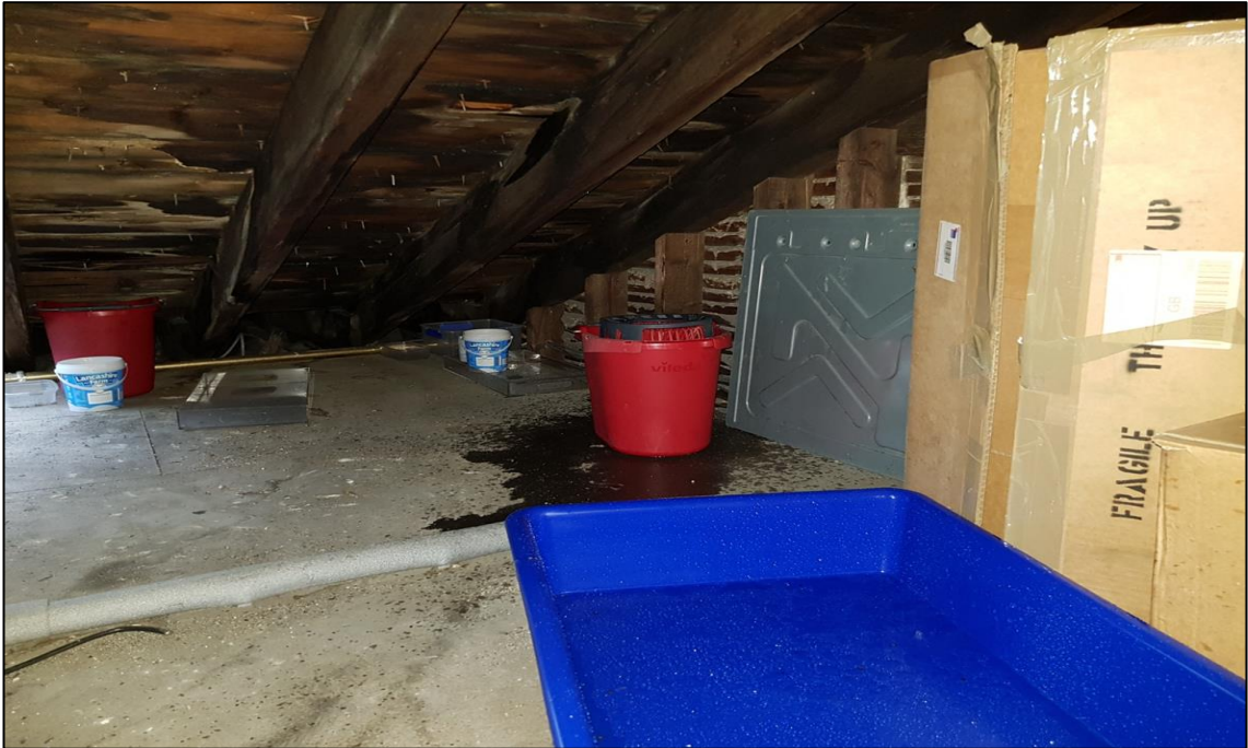
Figure 8 above: Buckets catching water from the leaking roof.
