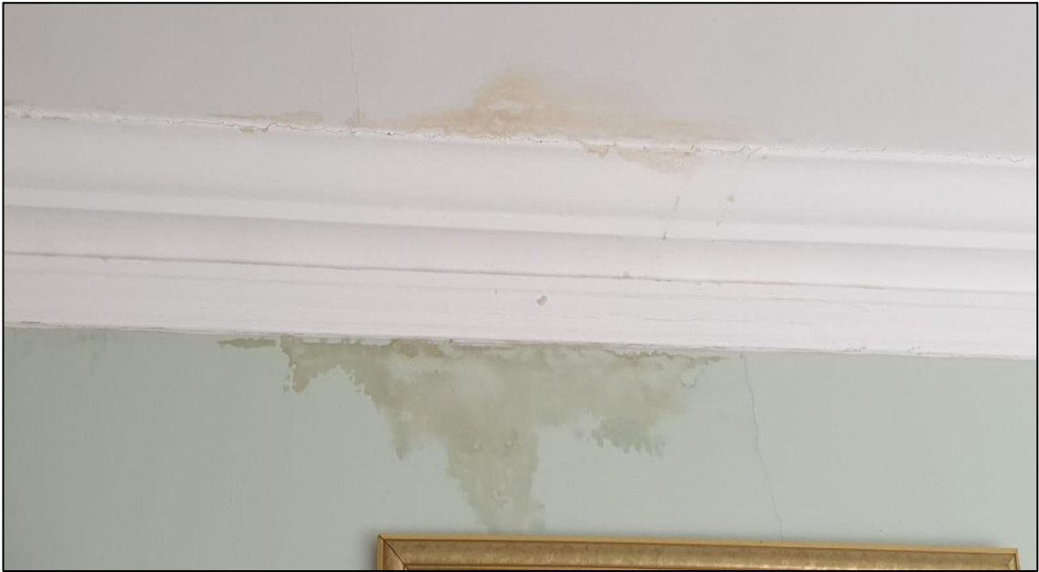
Figure 7 above: Water damage at 2F, 10 Randolph Crescent due to leaking roof.
