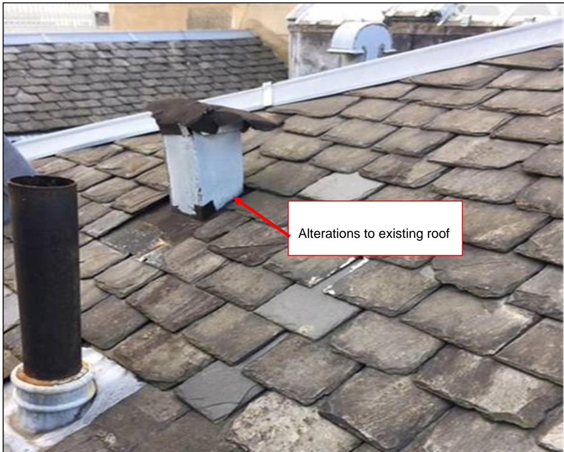
Figure 6 above: showing alterations to the existing chimney of no. 10 Randolph Crescent, noting further revisions to the existing roof.
